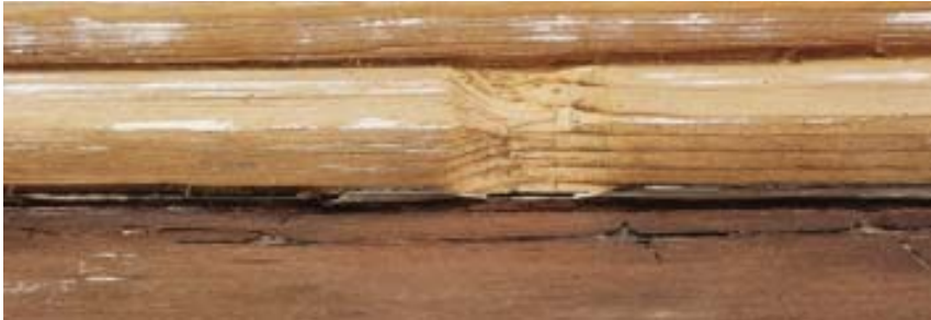
Figure 4. Finger joints on doors and windows are one place where rot can quickly gain a foothold, so the author creates a small recess with a utility knife and then skims over the joint with two-part epoxy putty to create a more water-resistant joint.
