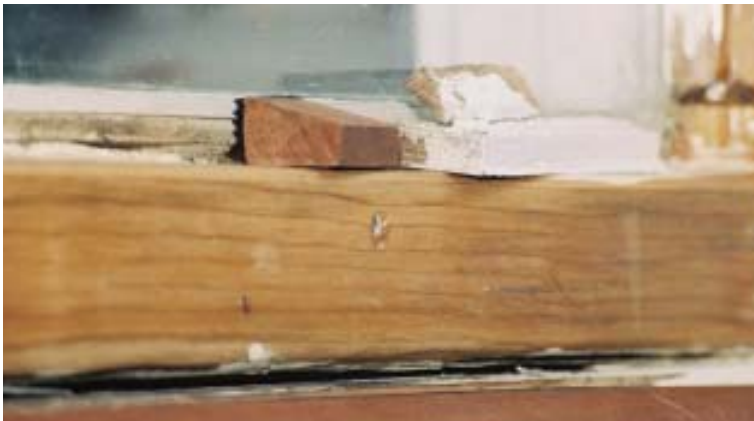
Figure 12. When the bottom stops on true-divided-light windows start showing the first signs of water damage, the author replaces them with wider versions cut from rot-resistant mahogany. Made with a steeper slope to aid in drainage, new stops are coated on all surfaces with two coats of epoxy. The black material on the front of the stop is a self-stick EPDM glazing gasket that the author uses instead of glazing putty.
