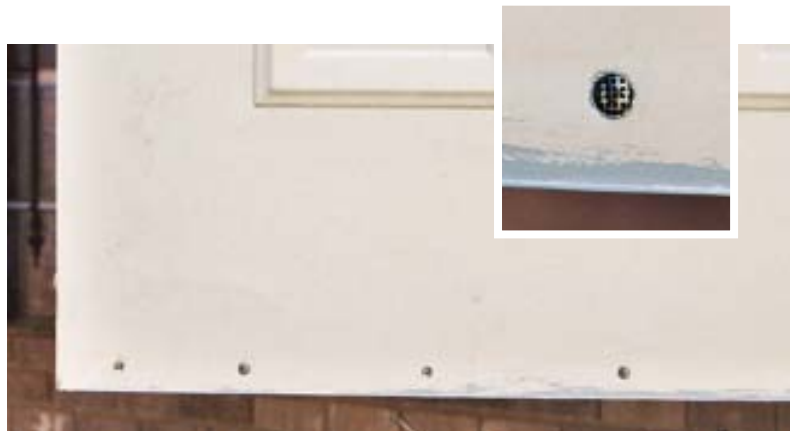
Figure 7. The wood bottoms on steel doors are vulnerable to rot. The author first removes the damaged wood and replaces it with pressure-treated stock, then drills a series of holes in the interior side of the door to promote drying. Small thimble vents inserted into these holes prevent insects from nesting inside the door.
