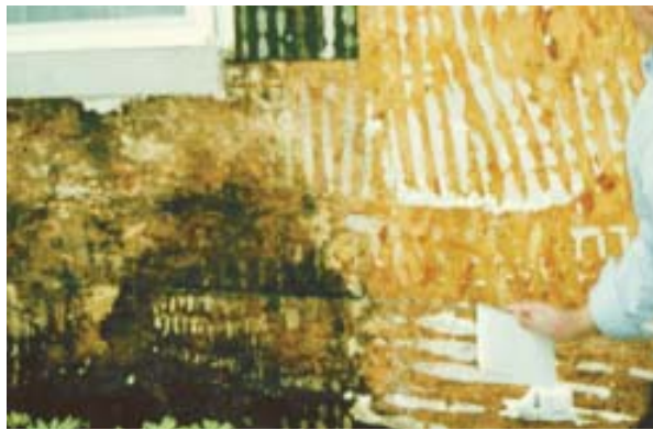
Figure 10. This wall shows characteristic damage from leaks at the window frame joints. Good flashings and a drainage plane would have saved the structure.
