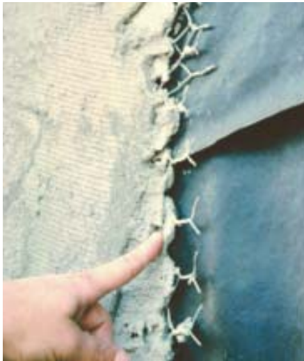
Figure 3. Portland cement stucco bonds tightly to modern asphalt felts, denying water the drainage space it needs to flow down and escape the wall. Moisture that penetrates stucco will saturate the paper and destroy its water repellency, wetting the wall structure beneath unless an air space is somehow created.
