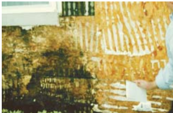
Figure 10. This wall shows characteristic damage from leaks at the window frame joints. Good flashings and a drainage plane would have saved the structure.
