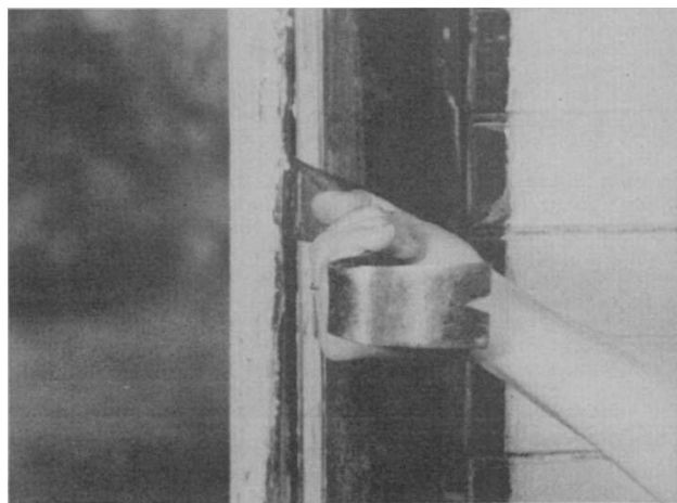
With a flat bar, pry off the parting bead to free the top sash.
