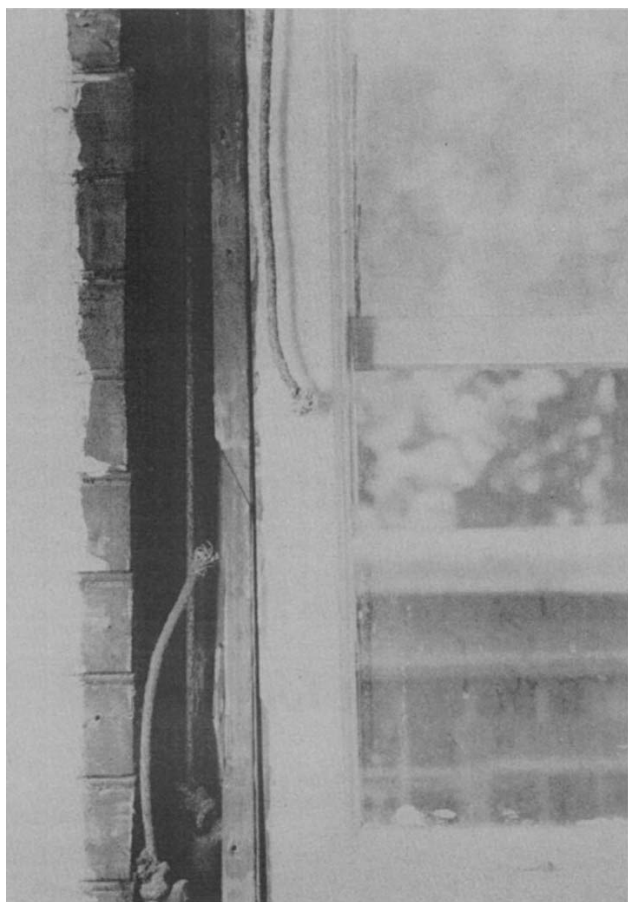
With the interior casing removed, the sash-cord weight is exposed. Spray foam can now be used to seal cracks around the window.
