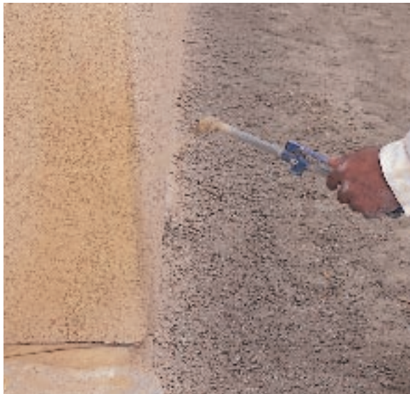
Figure 5. A fog coat can be brushed or rolled, but the author prefers to use a hand sprayer. Too much water will delay drying and darken the color, so use two thin coats instead of one thick coat, and feather the edges.
