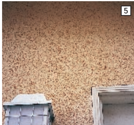
Figure 1. To patch a small crack (1), first mask both sides of the crack with tape, and dab the crack lightly using dry stucco on a small brush (2). To avoid ridges in the patch, brush off the excess (3), then remove the masking tape and brush again (4). Overnight condensation will provide enough moisture to cure the dry stucco and complete the patch (5).
