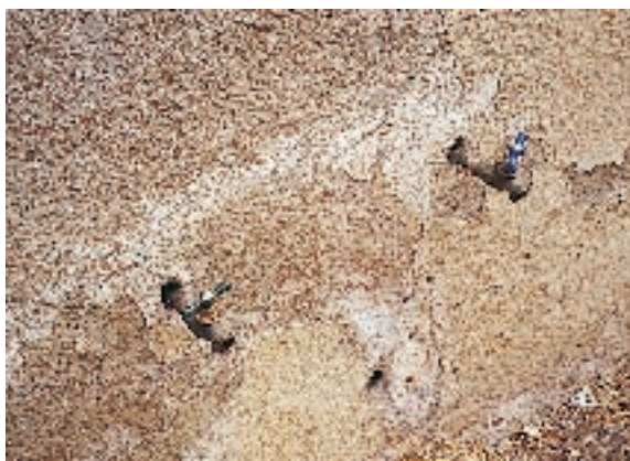
Figure 3. Scrape away efflorescence deposits with a wire brush, then saturate the surface with a 1-to-1 mix of vinegar and water. Flush with clean water before patching.
