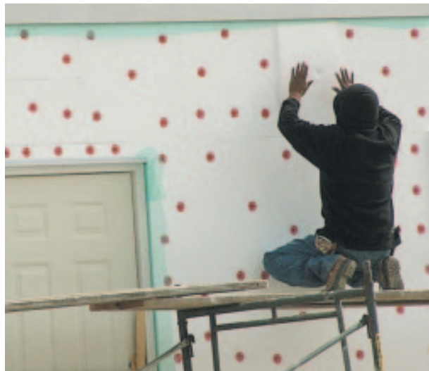
Figure 2. A worker attaches soft EPS "beadboard" with screws to form the base of the EIFS cladding. The close-up, below, shows the voids between the plastic beads. EPS allows water to leak through and can hold moisture against the building. That is why careful joint sealing and an effective secondary weather barrier are critical to system performance.
