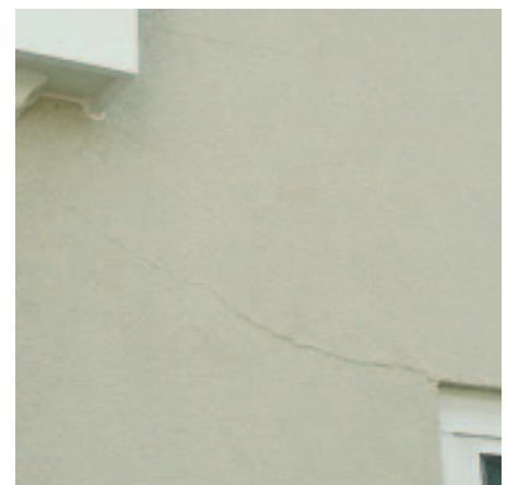
Figure 5. Window corners and narrow intersections between large wall sections are points of stress concentration where cracking may occur. If possible, the design should allow for isolation joints to relieve stress at such locations. In any case, the secondary weather barrier must provide protection for wall materials beneath the EIFS.
