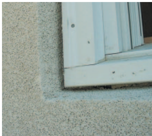
Figure 7. This joint between the EIFS and the brick-mold window casing should be sealed with backer rod and silicone sealant. Apply sealant to the base coat before the finish coat is applied. Be aware that many windows allow water to pass between the casing and the sill or jamb, so that surface joint sealing provides only partial protection. To protect the sheathing and framing, the secondary weather barrier and window flashing must be in place beneath the EIFS and the window.
