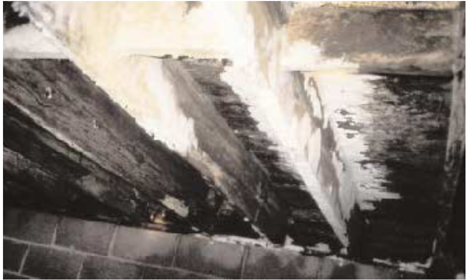
Figure 2. Trapped crawlspace moisture causes big problems as seen in this example where mold, mushrooms, and rot have overtaken joists and the underside of a subfloor.
