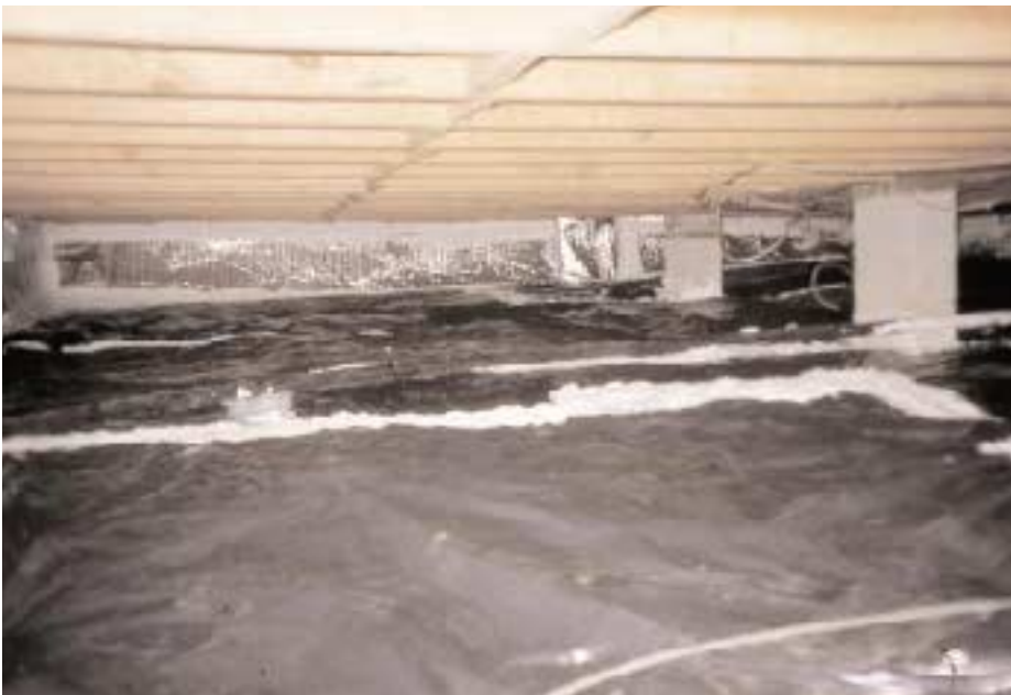
Figure 1. Crawlspace should be insulated and sealed shut, but only after they've been thoroughly dried out. This crawlspace has reflective wall insulation that is sealed where it meets floor plastic.
