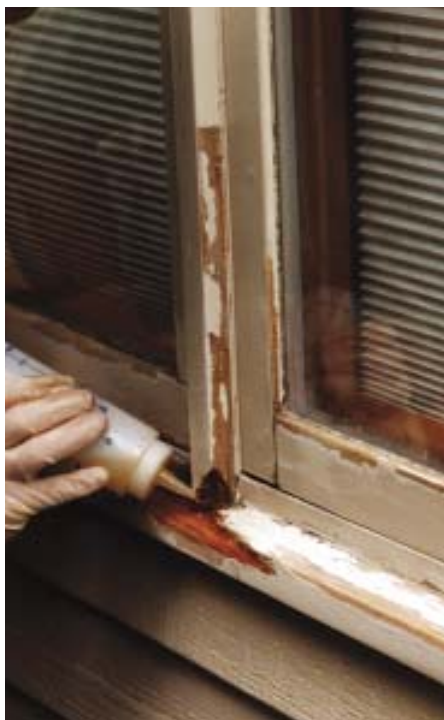
Figure 4. Rot damage needs to be repaired. Using liquid epoxy, the author saturates and consolidates areas that have minor rot (right). Where damage is more extensive, he first removes as much damaged wood as possible, then rebuilds the affected area with a two-part epoxy putty (far right and below).
