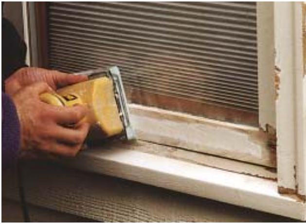
Figure 5. After the scraping and epoxy repair work, a palm sander loaded with 60-grit paper smooths the wood surface, feathering out the old paint and rounding over sharp edges. New unprimed windows should also be scuff-sanded to remove mill glaze.
