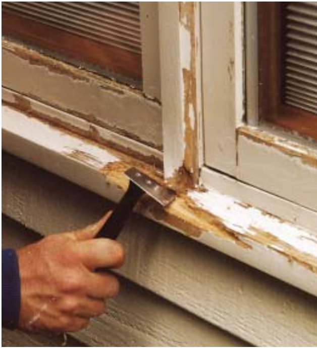
Figure 2. Scraping wood windows before they are repainted removes disbonded paint and reveals areas where rot has taken hold.
