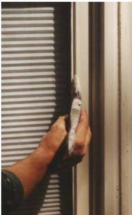
Figure 8. Using a 3 1 / 2 -inch angled sash brush, the author laps the paint slightly onto the glass, creating a final barrier against water intrusion.
