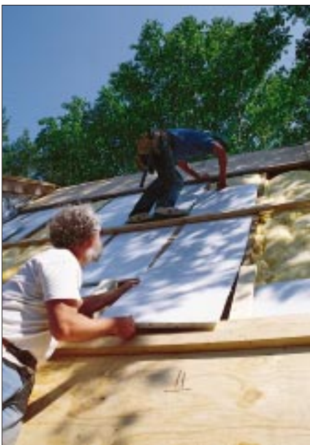
Figure 7. Two-by-four sleepers on top of existing rafters provide a ventilation chute beneath the plywood sheathing, while 1-inch rigid foam insulation prevents the fiberglass batts from expanding into the air space.
