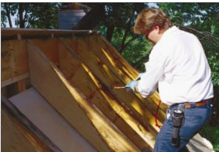
Figure 5. Before installing sister rafters and insulation, the existing framing was sprayed with a fungicide and insecticide.
