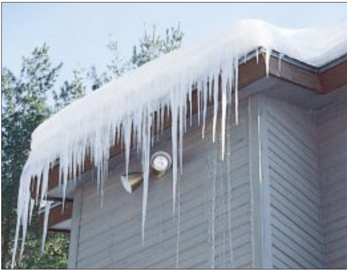
Figure 3. The winter before repairs were made, huge ice dams formed at the eaves of this cathedral roof. Water backed up into the soffits and walls, soaking interior and exterior finish materials.
