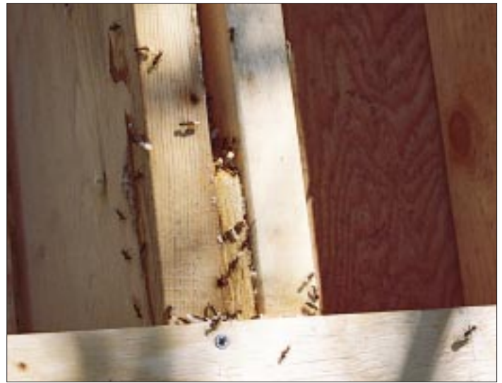
Figure 4. High moisture in the cathedral roofs created a perfect environment for carpenter ants, which tunneled into the insulation and nested in cracks between framing members.
